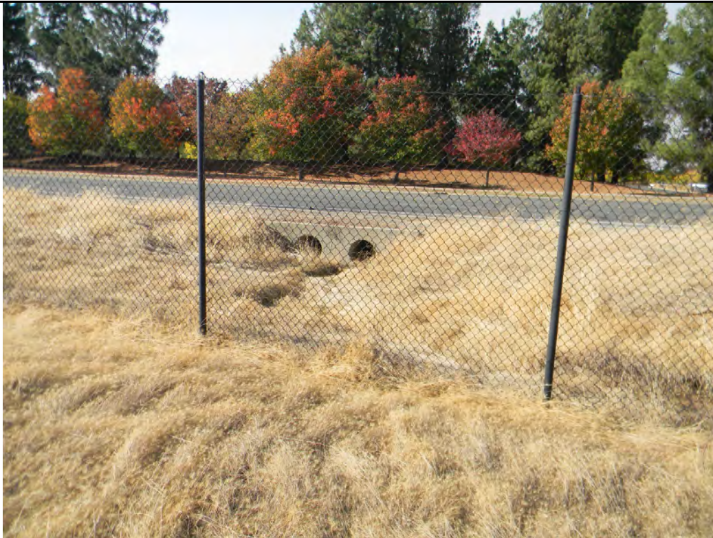
6. View to southwest at western property boundary, showing culverts where intermittent drainage (WS-1) passes under Foothills Blvd.
